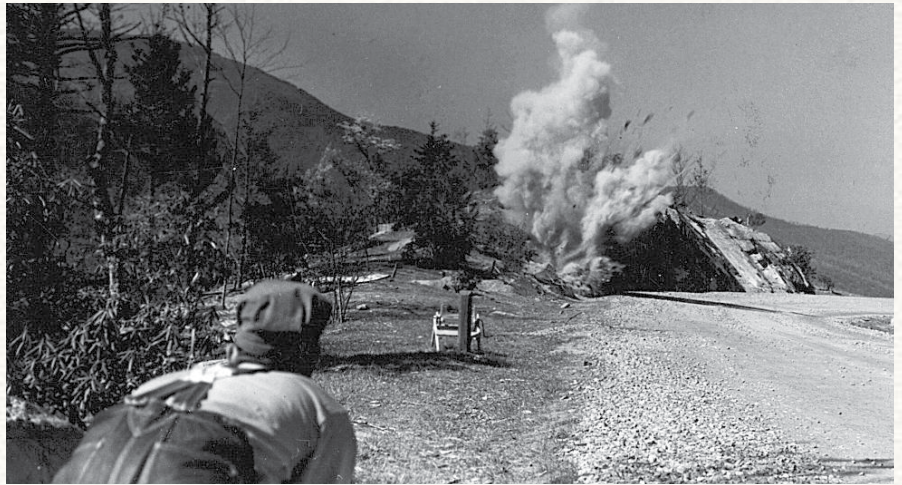
A worker monitors a dynamite blast during the early days of creating the Parkway.
